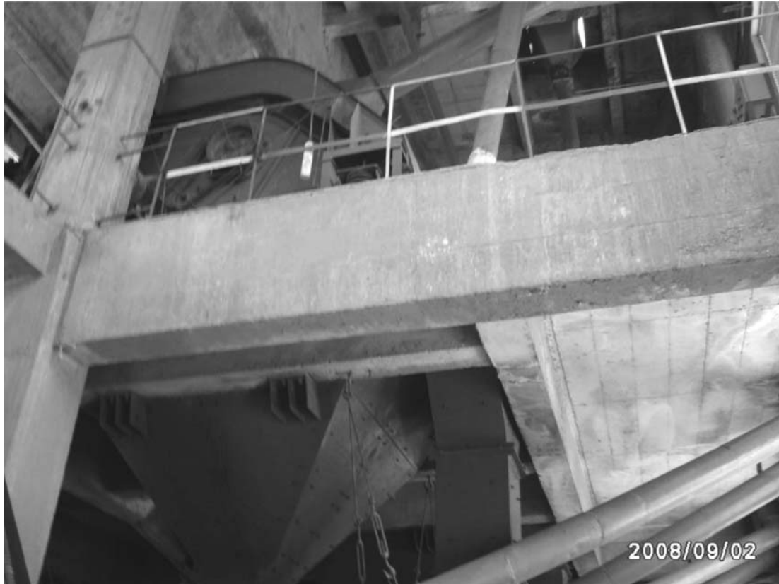
Figure 2.9: Wangji — Phosphate Plant Vibrating Screen
