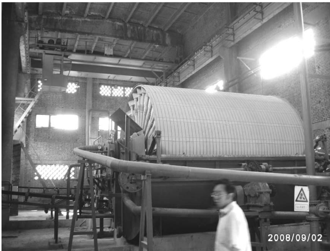
Figure 2.13: Wangji — Phosphate Concentrate Vacuum Drum Filter
