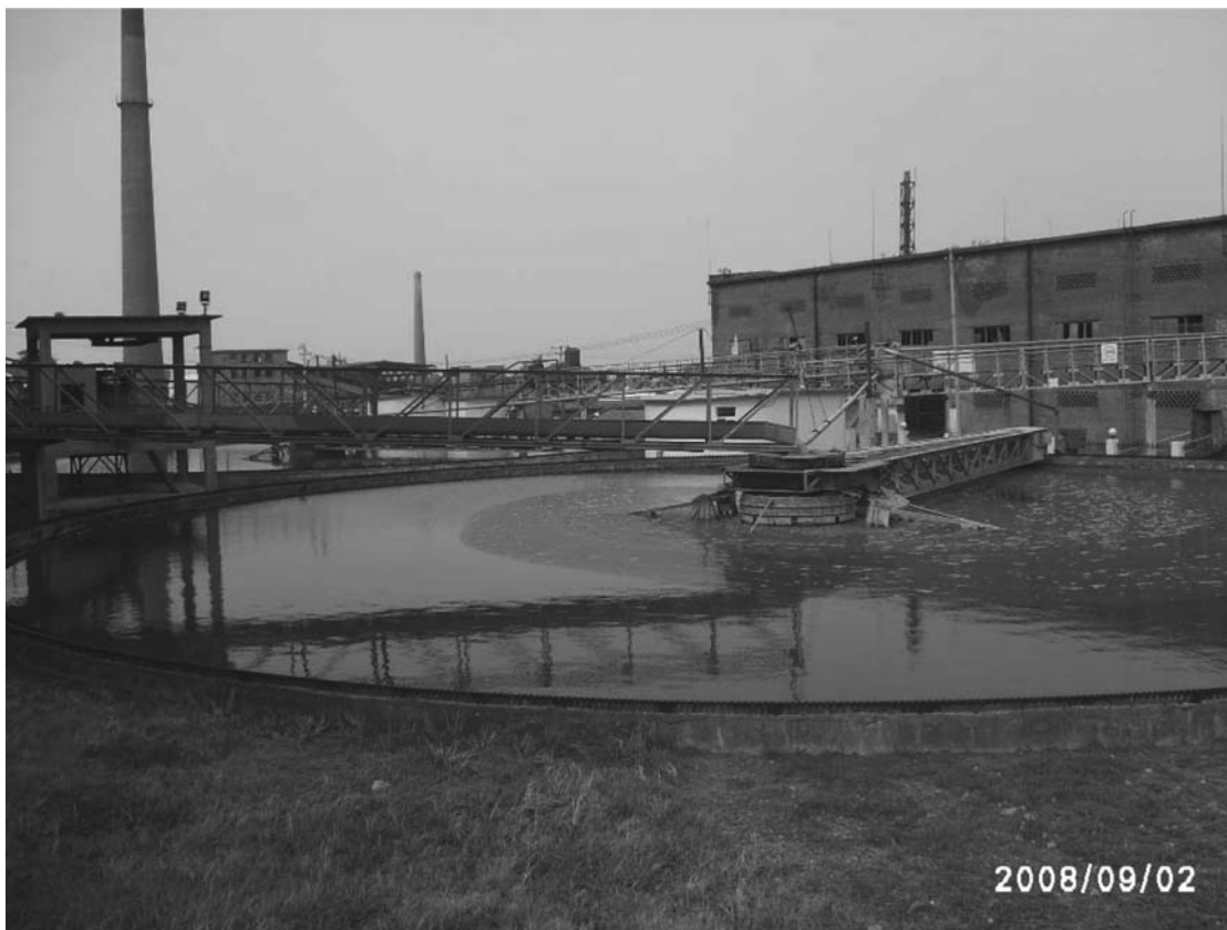
Figure 2.12: Wangji — Phosphate 45m Diameter Thickeners
