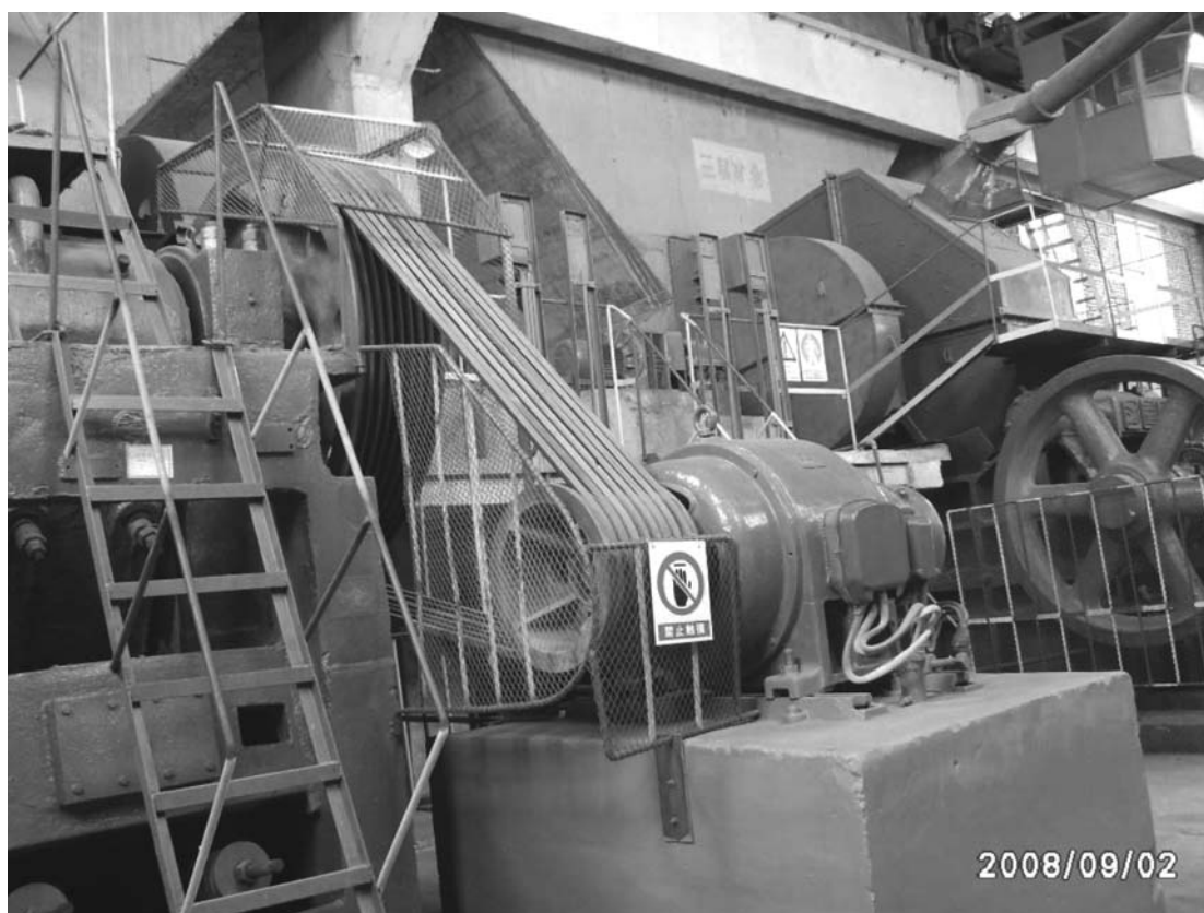
Figure 2.7: Wangji — Phosphate Plant Primary Jaw Crushers
