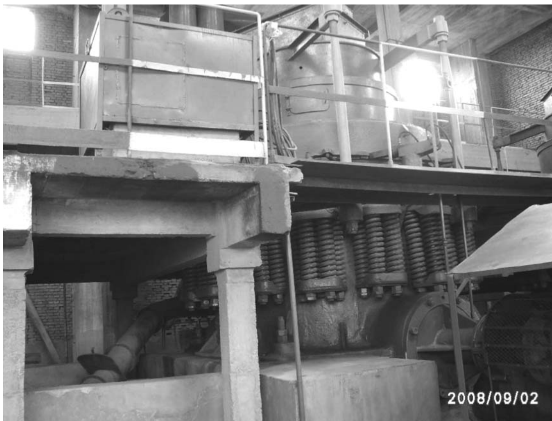
Figure 2.8: Wangji — Phosphate Plant Tertiary Cone Crusher
